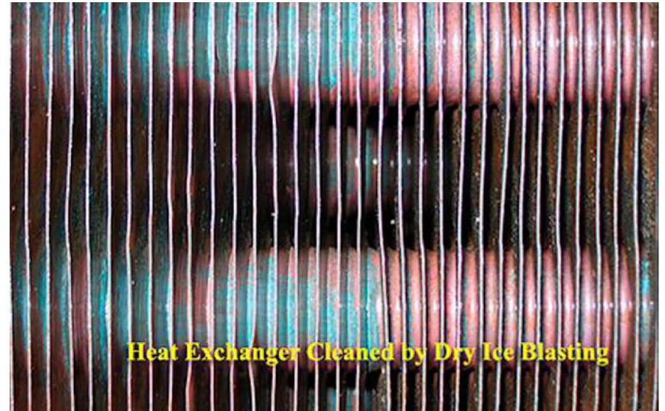
Heat Exchanger after
