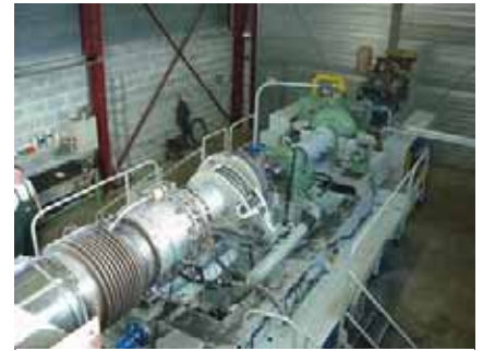
C40 being full load tested
