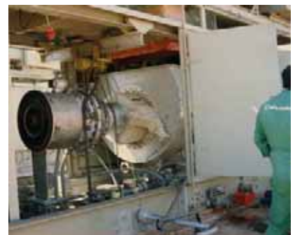
C40 engine under commissioning
