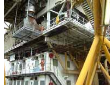
C50 GenSet on platform
